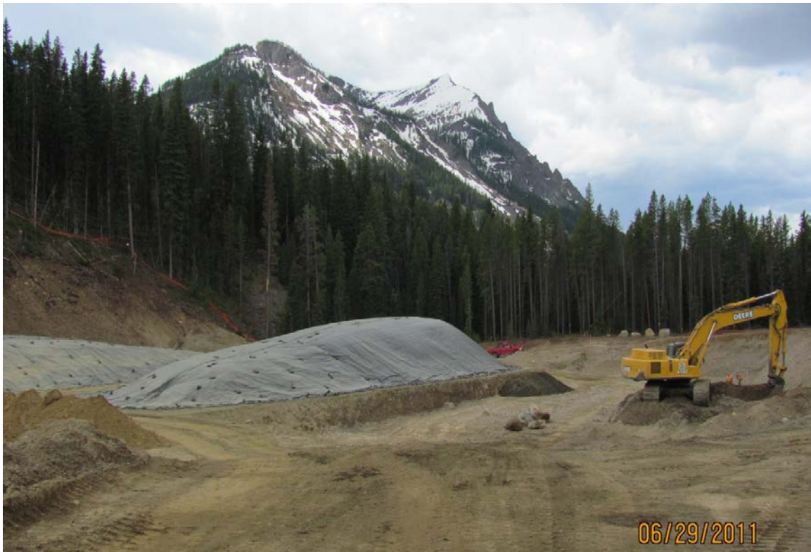
Figure 7. Construction of the repository at the McLaren Tailings site, note stockpiled and covered tailings pile to the left.
