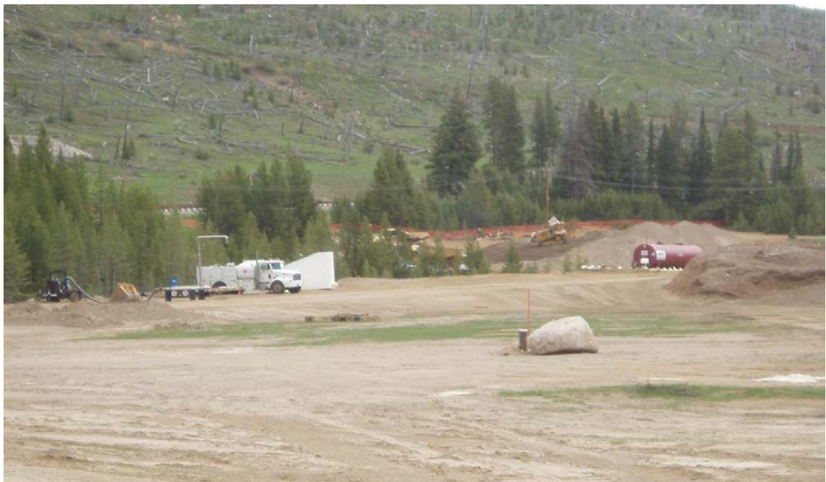
Figure 9. General tailings area at the McLaren Tailings site. Construction of the stream channel is in the far back, stockpiled cover soil is to the right behind and in front of the red fuel tank.
