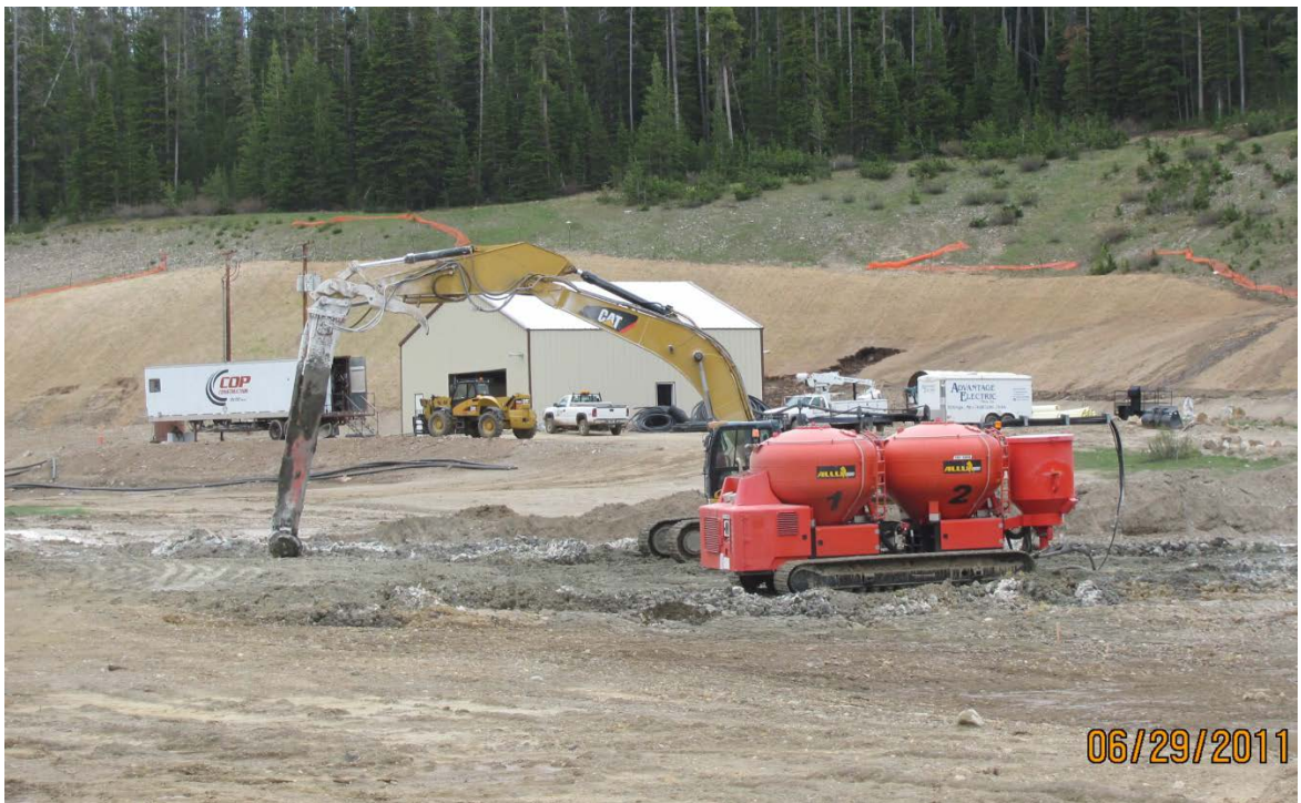
Figure 8. Lime mixing machine at the McLaren Tailings site. Lime is injected directly into the subsurface through the mixing head, a rotor tiller like machine attached to a track hoe. The mixing head is inserted into the tailings in an up and down motion to a depth of 22 feet evenly mixing lime with the pyritic tailings.
